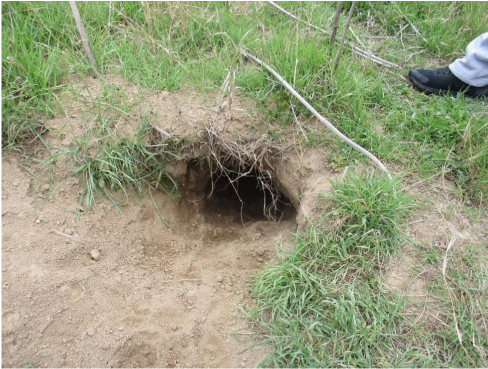
Photograph No 13: Hole near the embankment of Axios river
