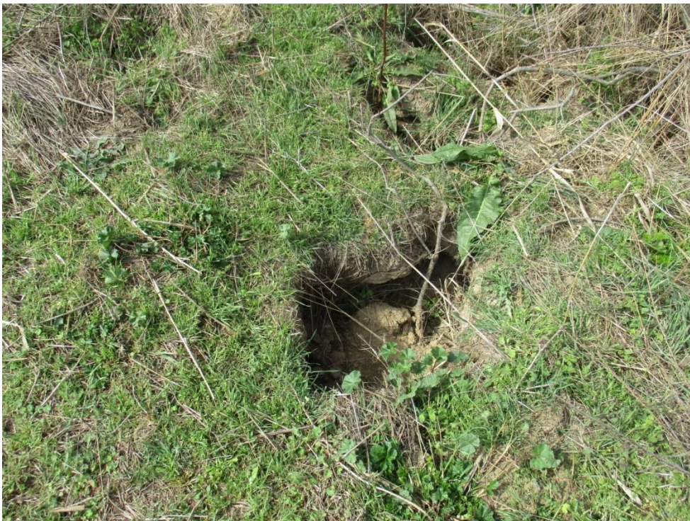
Photograph No 14: Hole near the embankment of Axios river
