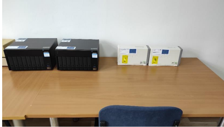
Figure 9: Uninterruptible Power Supply (UPS) and NAS Storage
